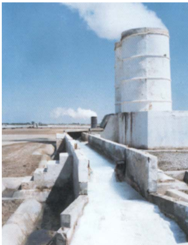
Figure 2 Deterioration by corrosion of brine conducting canals and silencer house built with reinforced concrete
