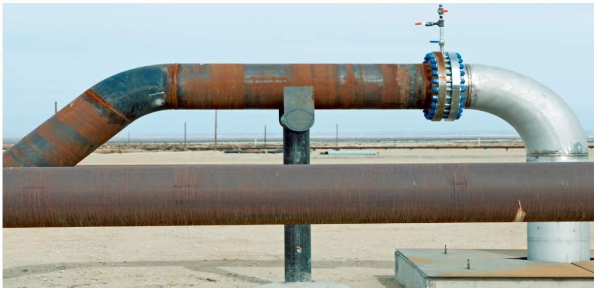
Picture 1-Uniform Corrosion of Pipelines
