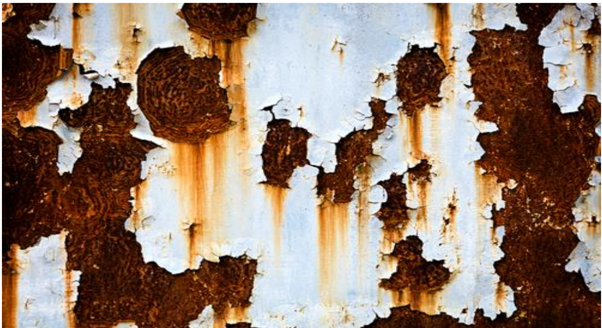
Picture 3-Filiform Corrosion on the surface of a pipeline
