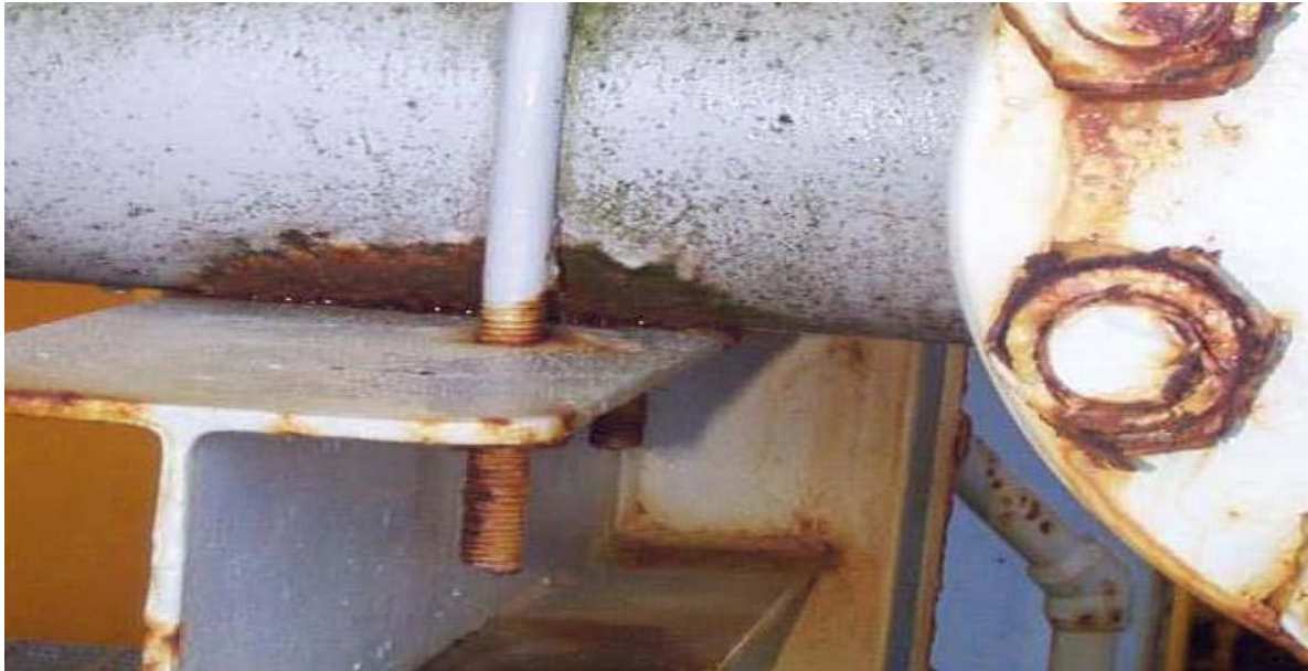
Picture 2-Crevice Corrosion of Pipeline
