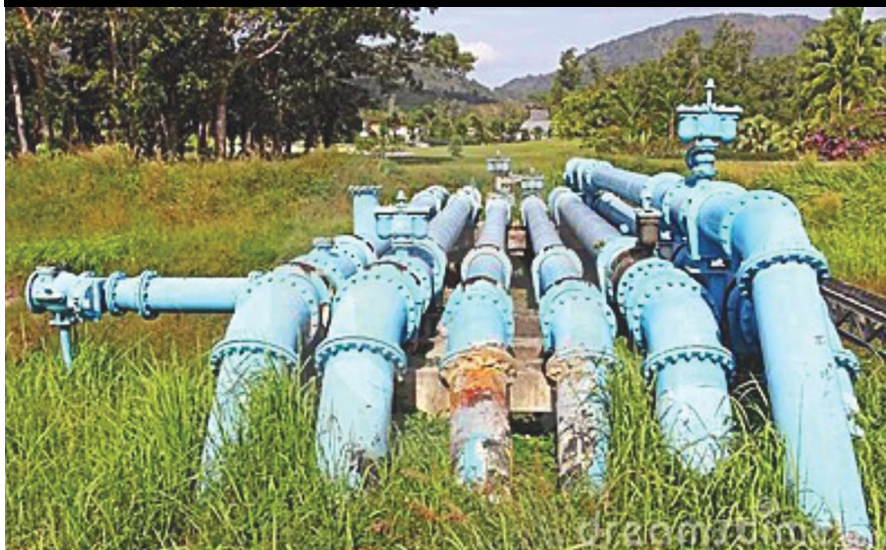
Painted steel water pipelines.
