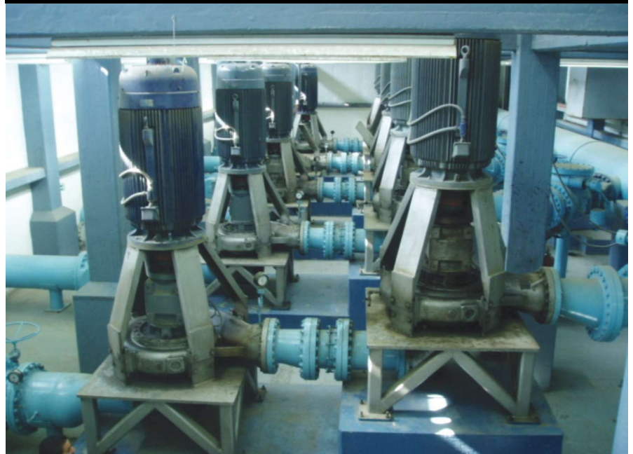
Pumps for water transportation.
