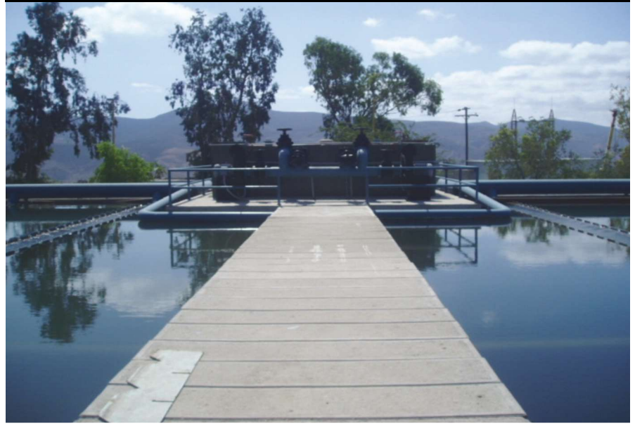
A plant for water treatment and clarification.
