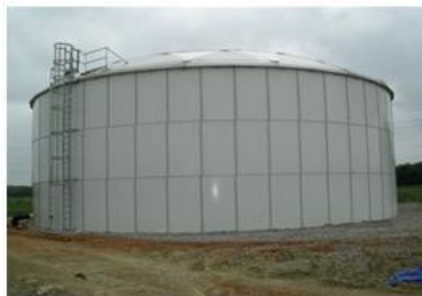
Figure 4: Fire protection water storage tank.
