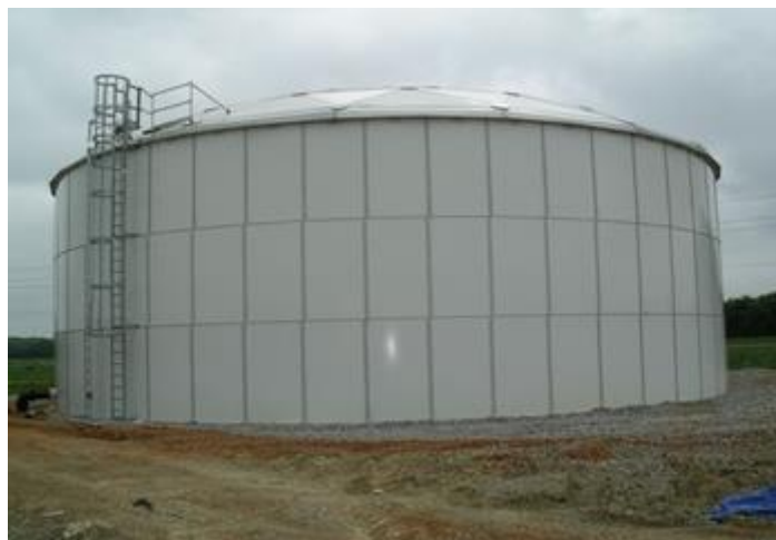
Figure 4. Fire protection water storage tank.
